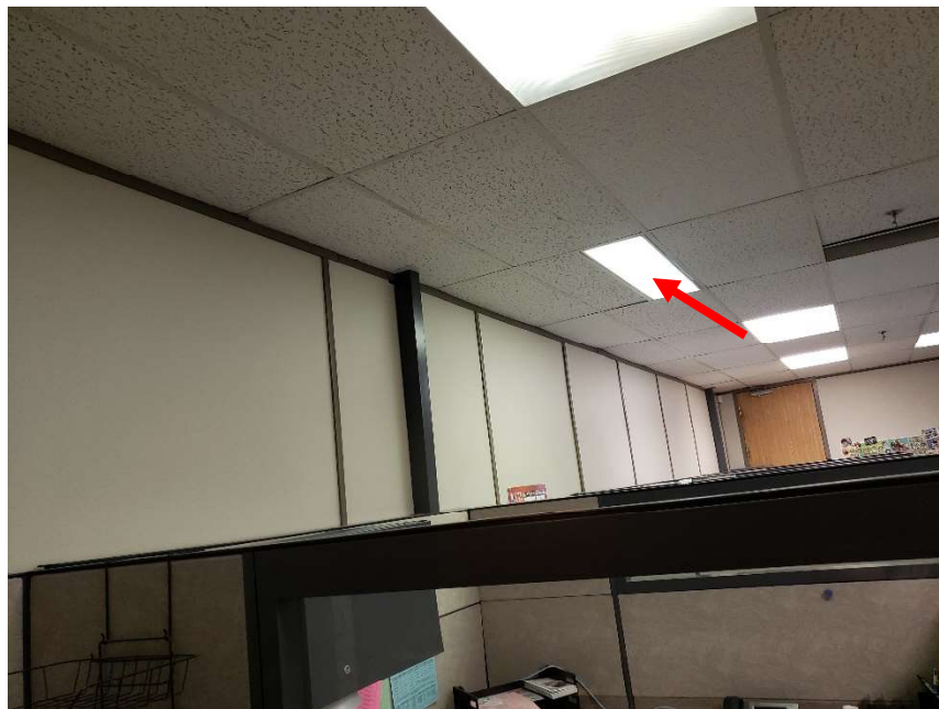
Photograph 4: Suspected mercury within light tubes throughout the Oral Health Administration Office.
