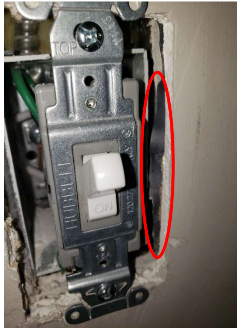
Photograph 1: Lead sheeting concealed behind drywall surfaces in the west and east partition walls in all four Operation Rooms and western Corridor located in the Oral Health Clinic.
