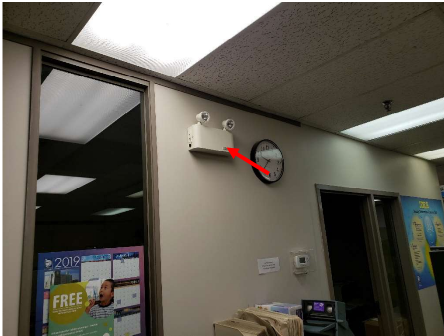
Photograph 3: Presumed lead-containing batteries within emergency lighting.
