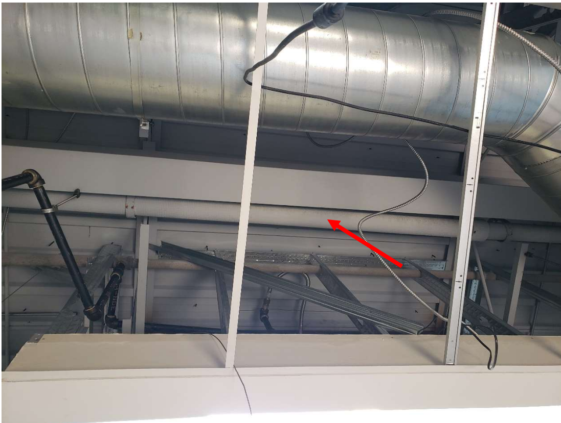
Photograph 6: Asbestos-cement (also known by the tradename Transite™) observed in the traversing ceiling space throughout the Unit.
