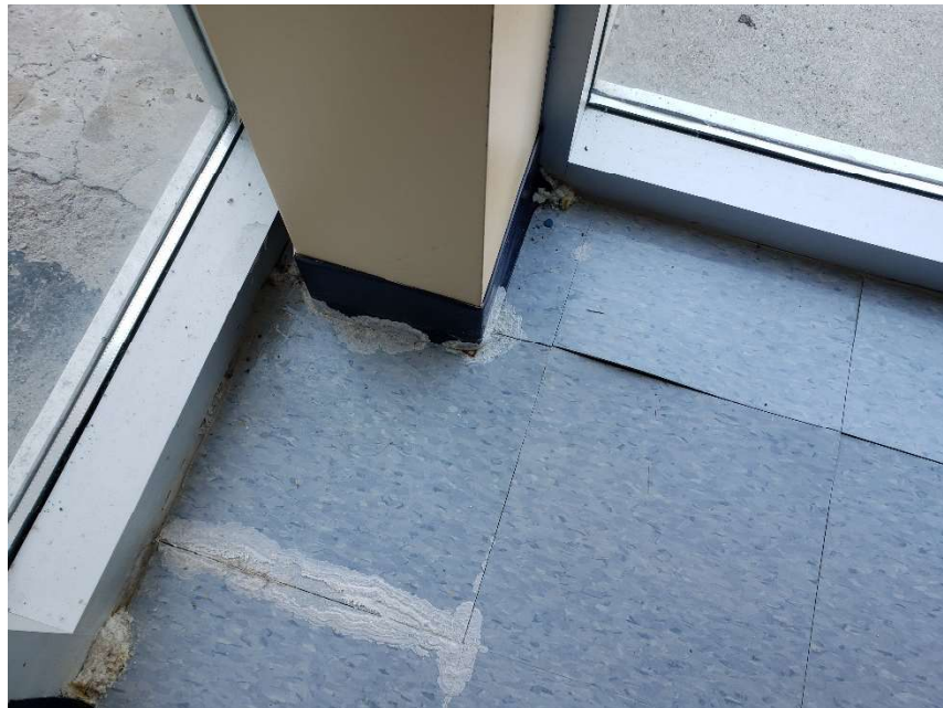
Photograph 4: Water-damaged non-asbestos vinyl floor tiles and drywall.
