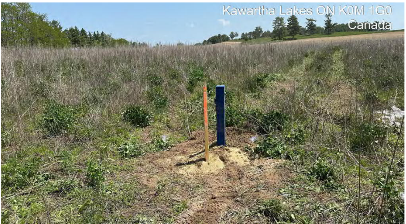
Photograph #4 – Looking east. Monitoring well is installed in the area of the proposed underground water storage tanks (Borehole FST-01).
