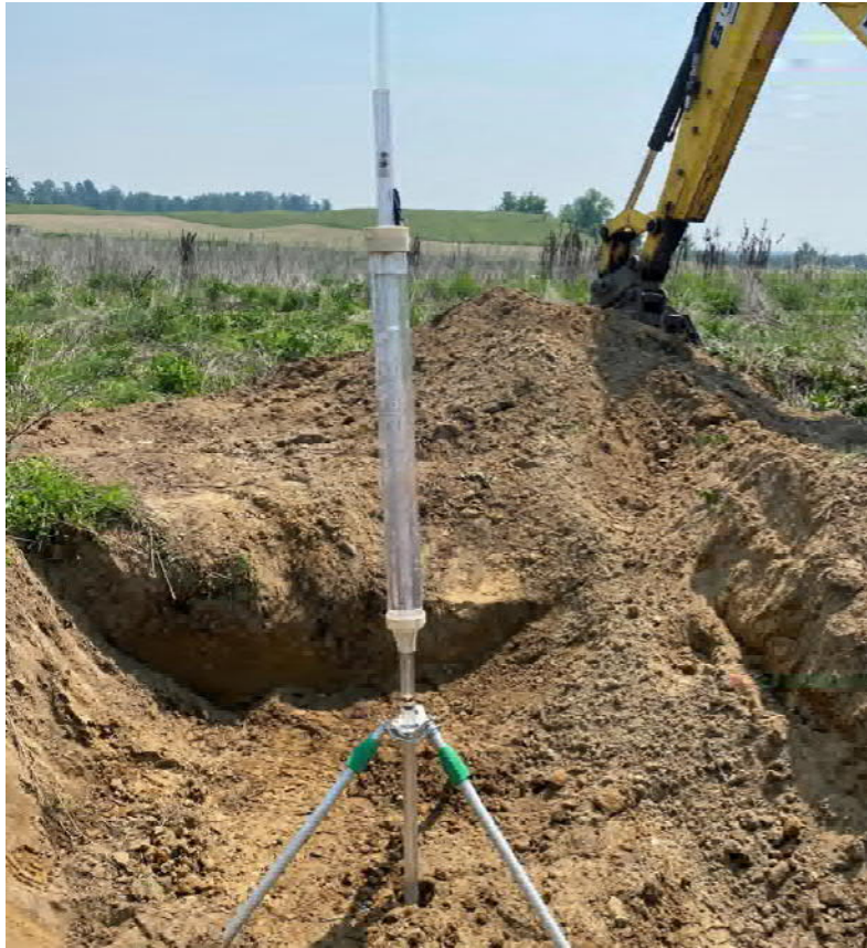
Photograph #5 – Test pit excavation to perform in-situ infiltration (Guelph permeameter) test at the proposed stormwater management pond location (Test Pit TP-01).
