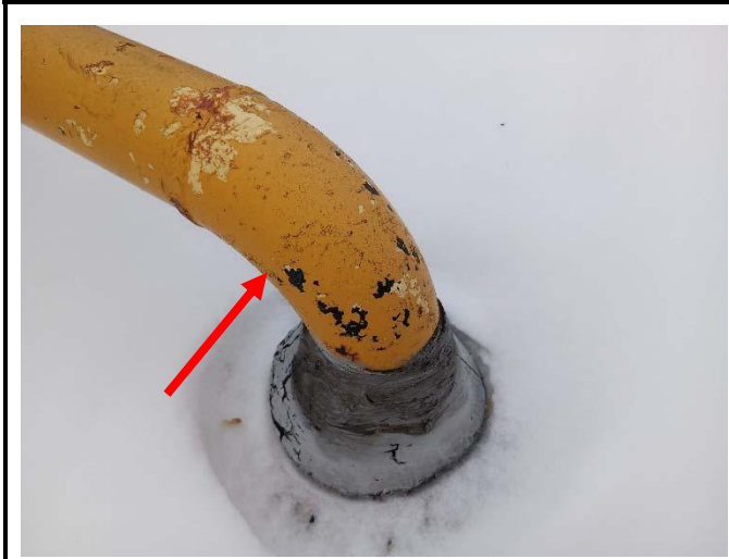
Photo 1: View of the lead containing yellow paint (see arrow) observed to be in fair condition on the metal roof piping.
