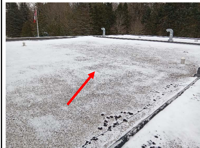
Photo 3: View of the presumed asbestos containing built-up roofing (see arrow) observed on the Roof of the Subject Building.
