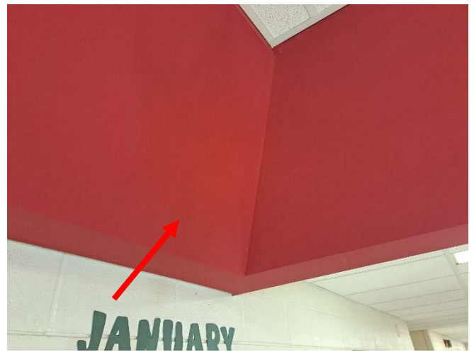
Photo 2: View of the lead containing red paint (see arrow) observed to be in good condition on the bulkhead in the Main Foyer.
