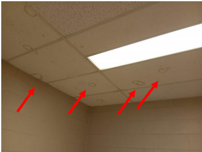
Photo 3: View of the apparent water stains (see arrows) observed on six lay-in acoustic ceiling tiles within the Boy's Changeroom 138.
