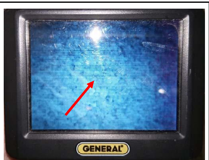
Photo 6: View of exterior facing wall cavity (see arrow) observed with a borescope indicating no presence of vermiculite within Custodian Room 130 of the Subject Building.
