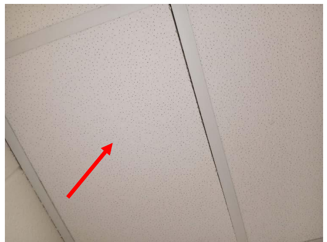
Photo 4: View of the non-asbestos containing white 4' x 2' textured acoustic ceiling tiles with pinholes (see arrow) observed within the Corridor 107 near the Main Foyer.
