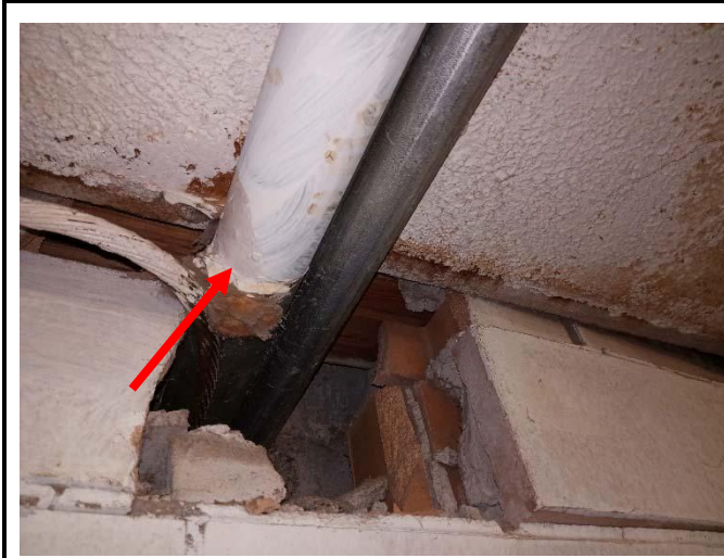
Photo 9: View of non-asbestos containing fibreglass pipe insulation (see arrow) observed in Custodial Room 147 within the Subject Building.
