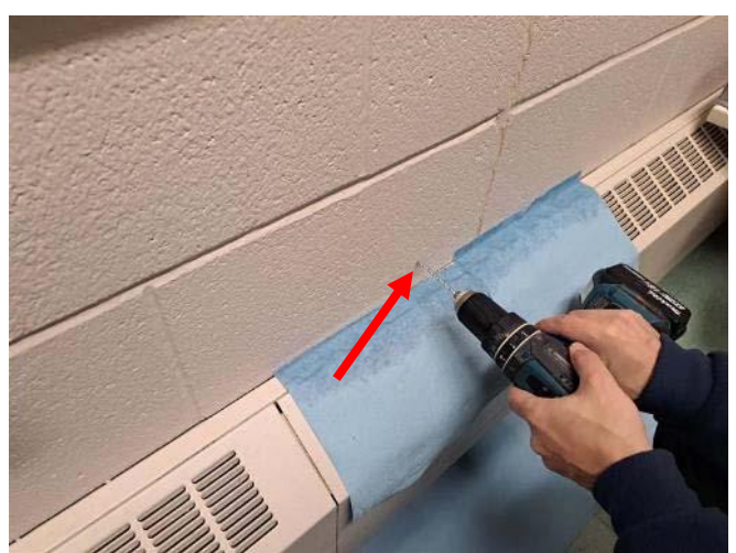
Photo 4: View of the interior wall during the vermiculite investigation and drilling activities prior to repair patching (see arrow) within Room 109 of the Subject Building.
