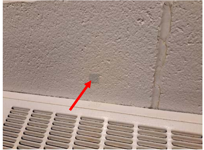
Photo 6: View of the interior wall post vermiculite investigation and drilling/ patching activities (see arrow) within Room 109 of the Subject Building.
