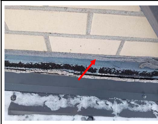
Photo 1: View of the asbestos containing grey caulking (see arrow) observed to be in poor to fair condition on the Roof Flashings of the Foyer Roof.
