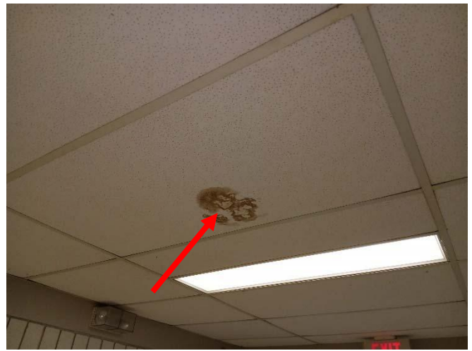
Photo 10: A view of water-staining and suspect mould (see arrow) observed on non-asbestos containing acoustic ceiling tile in Corridor 172 within the Subject Building.
