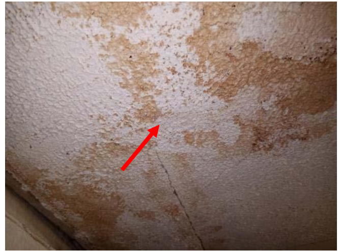
Photo 2: View of the ceiling finishes with associated non-asbestos containing white compound (see arrow) observed to be water-stained in Custodial Room 147 within the Subject Building.
