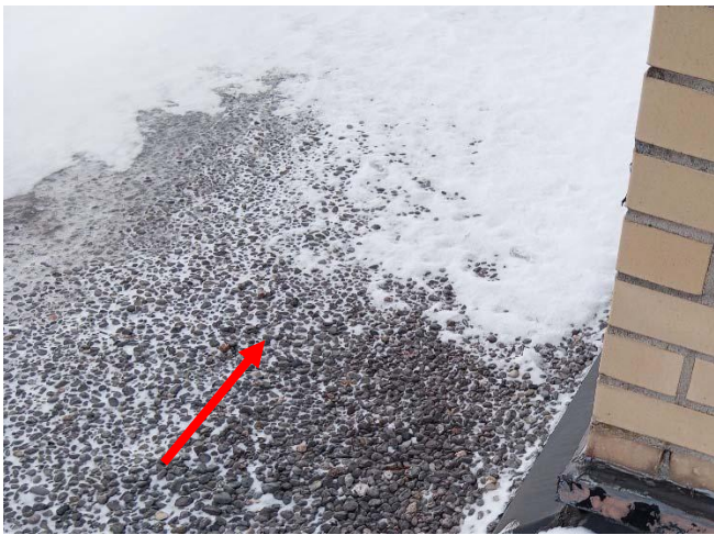
Photo 7: A view of the built-up roofing system (see arrow) observed throughout the Roof of the Subject building.
