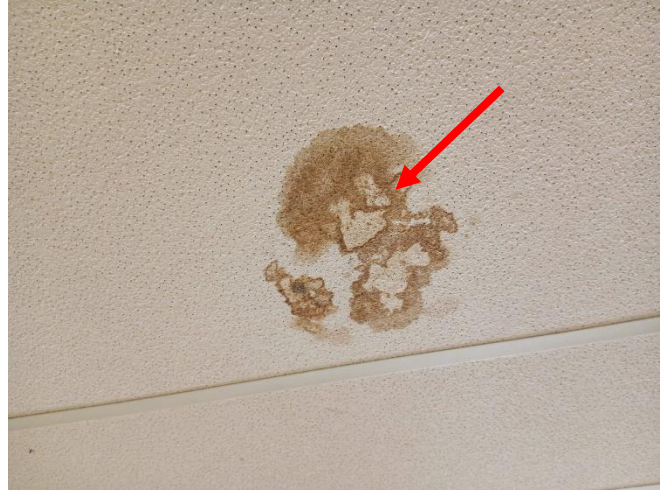
Photo 2: View of the visual suspected mould growth (see arrow) observed on lay-in acoustic ceiling tiles within Corridor 159A.
