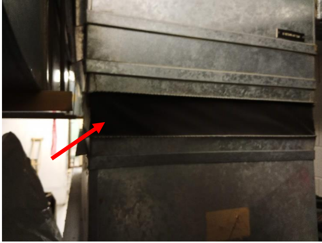
Photo 1: View of presumed asbestos containing vibration dampers (see arrow) observed to be in good condition within Boiler Room 141.
