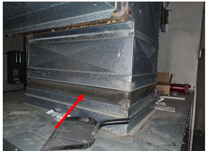
Photo 8: View of a presumed asbestos containing vibration dampener in Mechanical Room 201 within the Subject Building.
