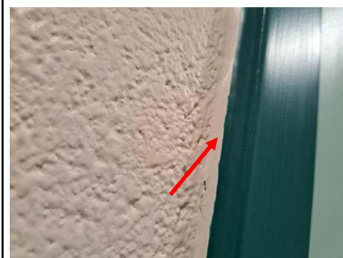
Photo 3: View of the asbestos containing beige caulking (see arrow) observed to be in good condition on the door frames within Rooms 108 and 109 of the Subject Building.
