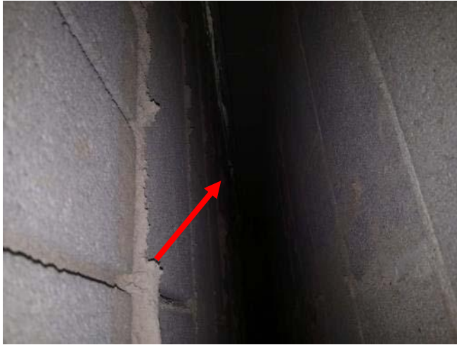
Photo 5: View of the void wall cavity (see arrow) observed during the vermiculite investigation between Room 108 and Room 109 of the Subject Building.
